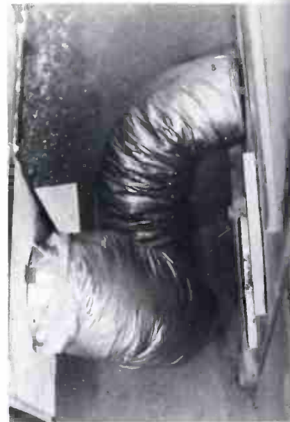
Looking down at transmitter from above; fresh air duct at left
